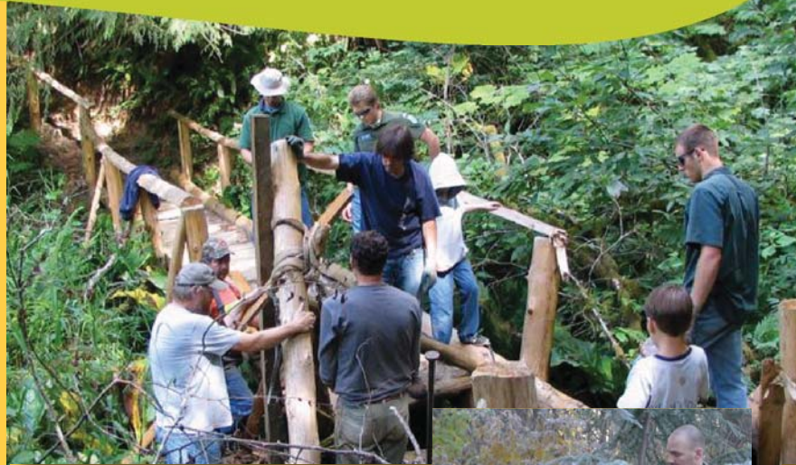
Above, a team coordinated by Friends of Schafer & Lake Sylvia State Parks (FOSLS) works on repairing a bridge at Lake Sylvia. Grays Harbor Stream Team events at Alder Creek and Lake Sylvia provided fun activities for all ages.
